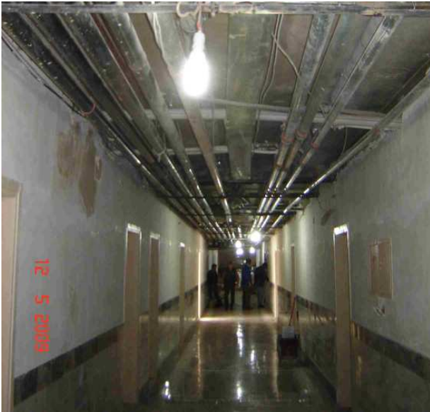
Before: Internal pipes-no insulation
