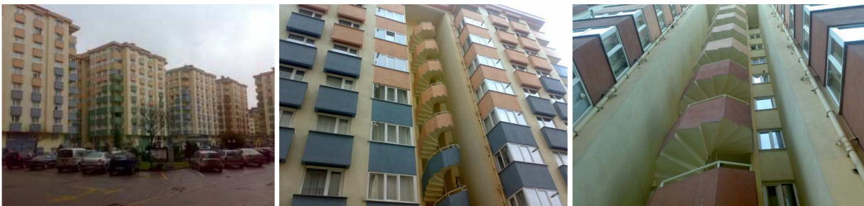
Apartment Complex upgraded to RE27 with MULTICERAMICS color matched to original painting.
